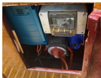
Shore Power Connector Master Battery Switch Battery Loading
