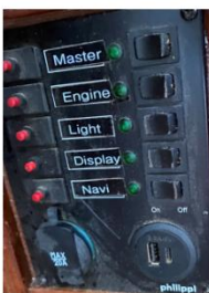
Master switch board
